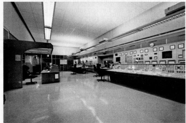
One of the two control rooms, controlling generators 1 and 2 which are the older pair. The control room is sited between the two generator halls.
